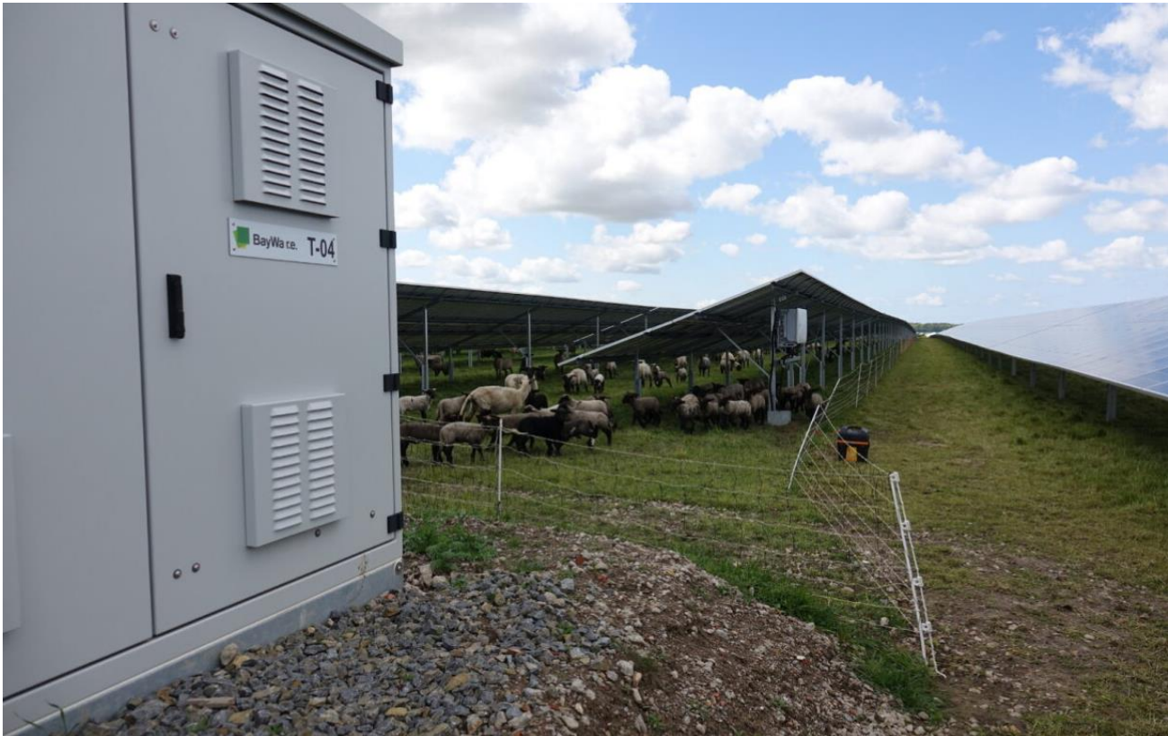
Plate 3: Typical transformer on a solar farm site
